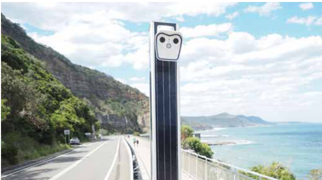
Camera incident detection facilities in NSW offering minimised camera deflection in high wind areas.
