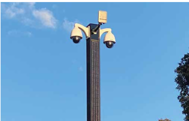
On campus security with dual camera and communications at UOW.
