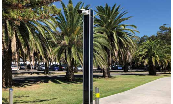
Marina park safety infrastructure using PowerStack in Australia.
